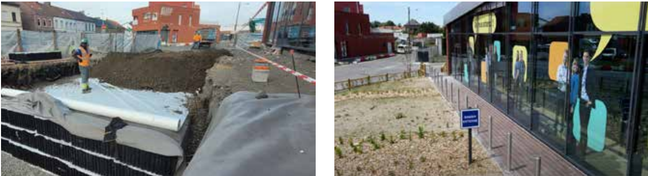
300M 3 - VIEUX CONDÉ Rainwater runoff from the roof and car park was taken into account during the construction of this new LIDL supermarket. This collection basin allows for temporary stormwater storage, before gradually allowing said water to infiltrate.
