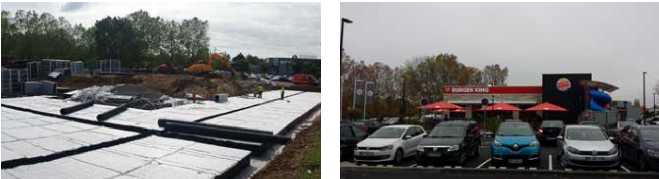
1,250M 3 - LABÈGE To reduce the impact of this new construction and limit rainwater runoff, an underground Nidaflow basin can store nearly 1200 m 3 of water. It thus prevents water systems from overloading during heavy rains, and limits flood risks.
